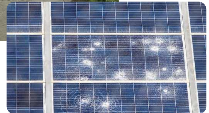
Solar panels damaged by hail ( aviva.co.uk )
